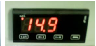
Controller and Temperature display
